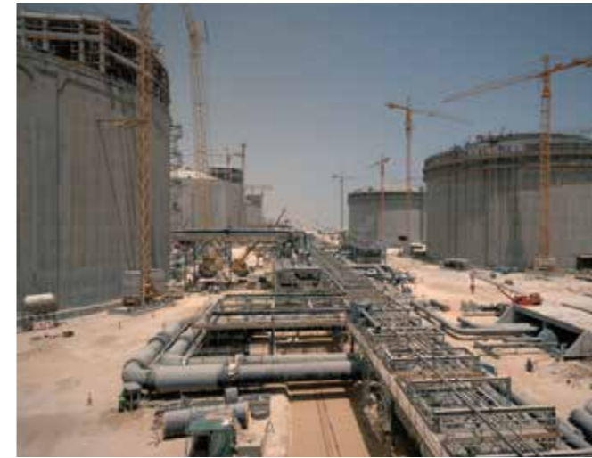
Gor Gas Project, Western Australia
